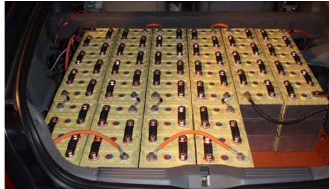
Figure 5 Battery pack in an electric car showing 64 of the 100 batteries in the pack
